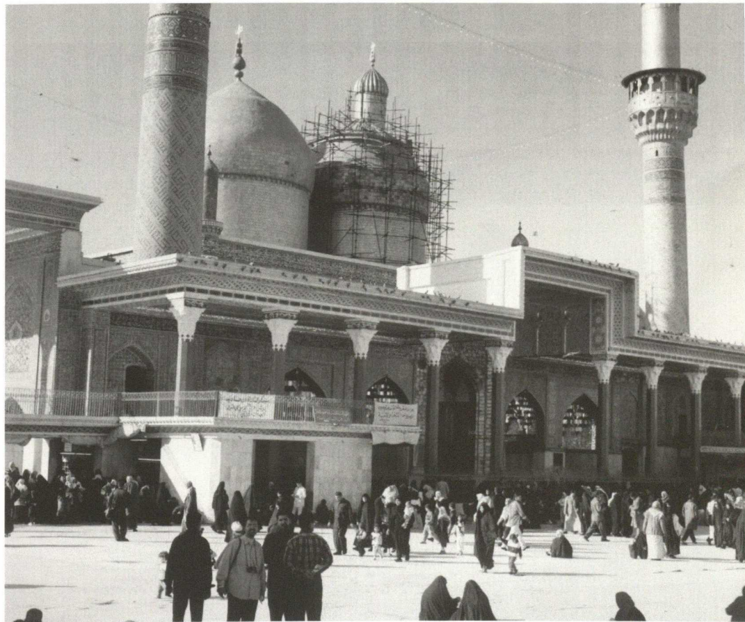
Inner courtyard of the Kazimain Mosque in Baghdad, one dome in the process of receiving a new gold coating
