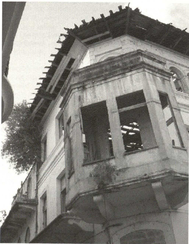
Mansion Obarrio, historic centre. World Heritage (aggressive biological attack on the structure, Nov. 2002).
