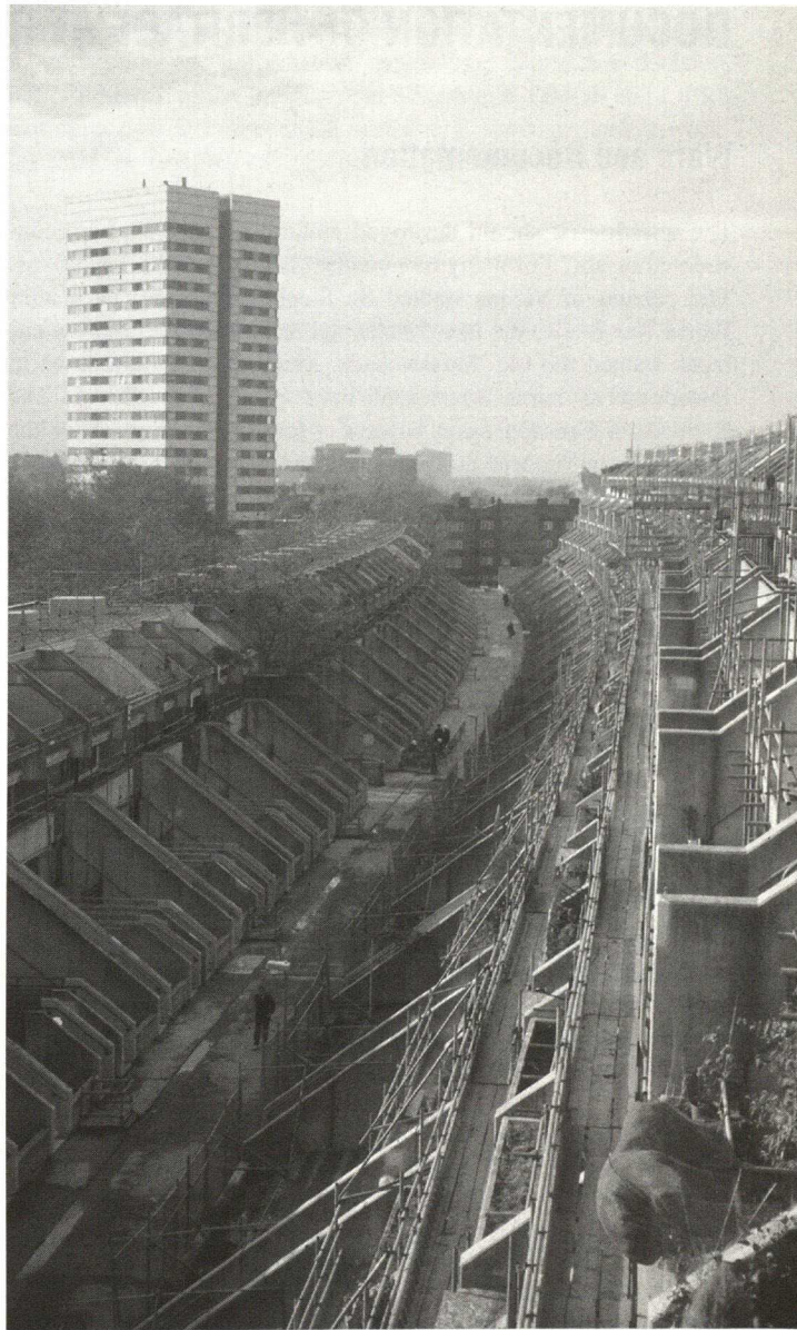
The Alexandra Road Housing Estate in London during the large-scale concrete repair programme in 1998. Attempts to rectify earlier poor repairs and address later problems were difficult to carry out without resulting in a blotchy looking building instead of the sleek, high quality concrete finish of the original concrete. (Photo: S. Macdonald)
