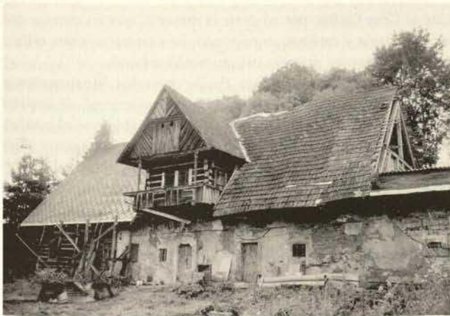
Havlovice, land-register No. 36, District of Trutnov - a timbered farm from the end of the 18th century in a critical state
