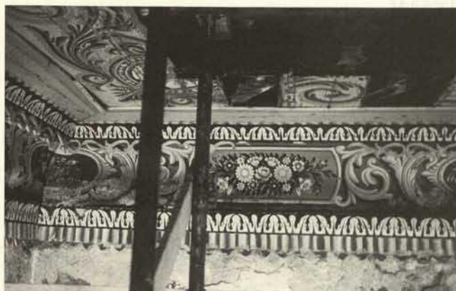
Akko, historic town, decay of decorated ceilings
