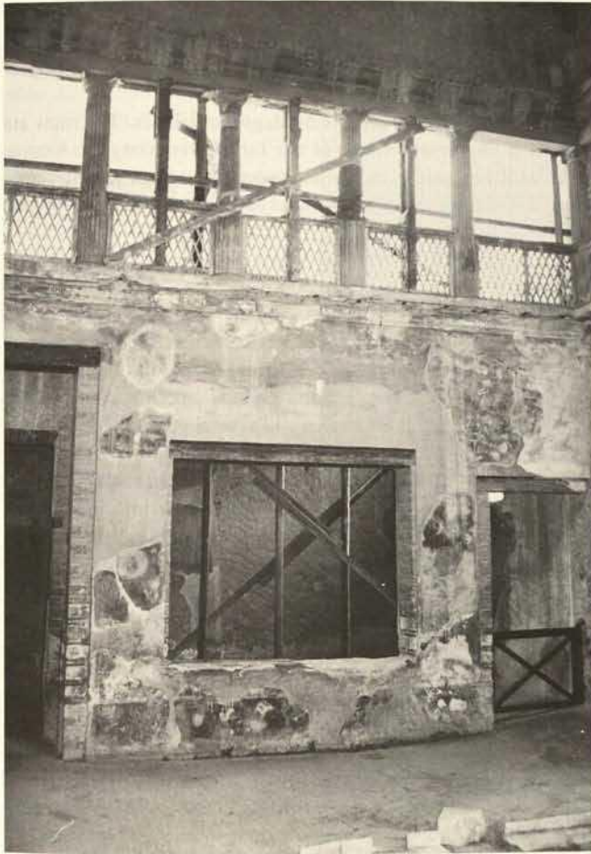
Casa sannitica: provisionally supported ceilings and severe water damages due to leaking roof
