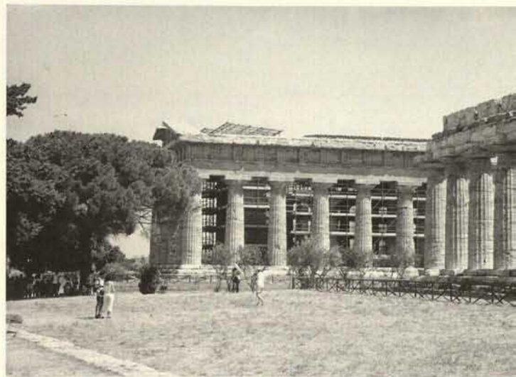
Paestum, "Tempio di Nettuno", interior still in scaffolding, and Basilica with protective fence
