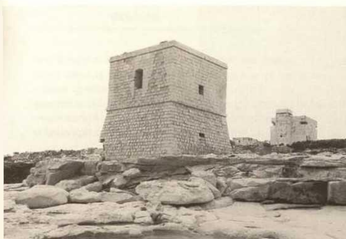
Coastal tower (c. 1658/59), damaged by natural processes
