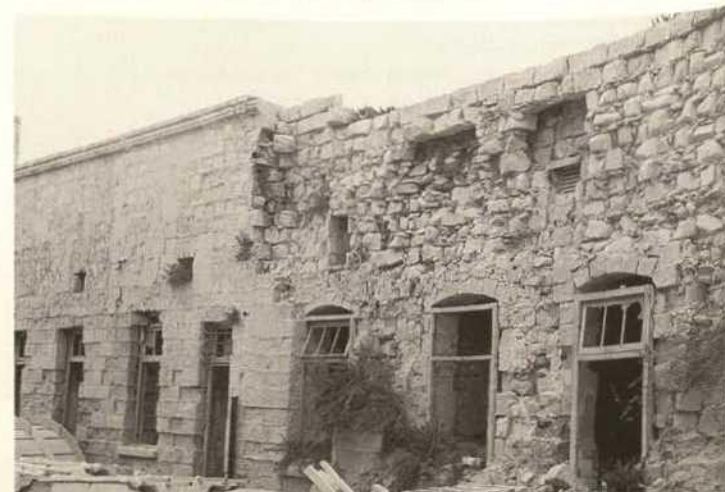
Fort Ricasoli (1670-1900), severely damaged magazines
