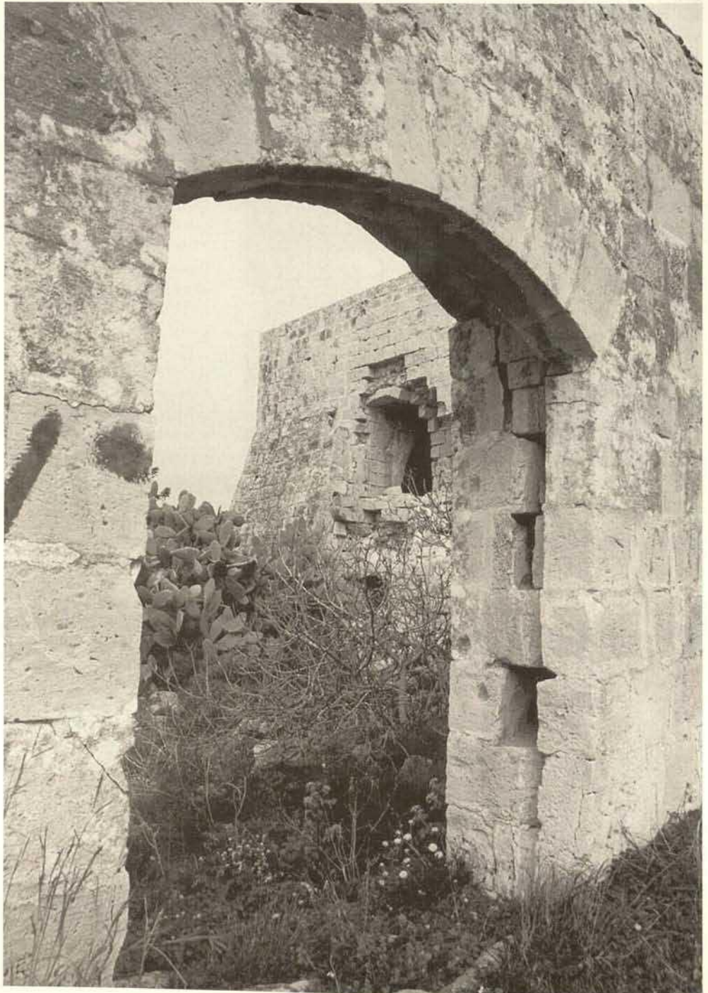
Casa Ippolito (1664), abandoned and severe structural damage in parts
