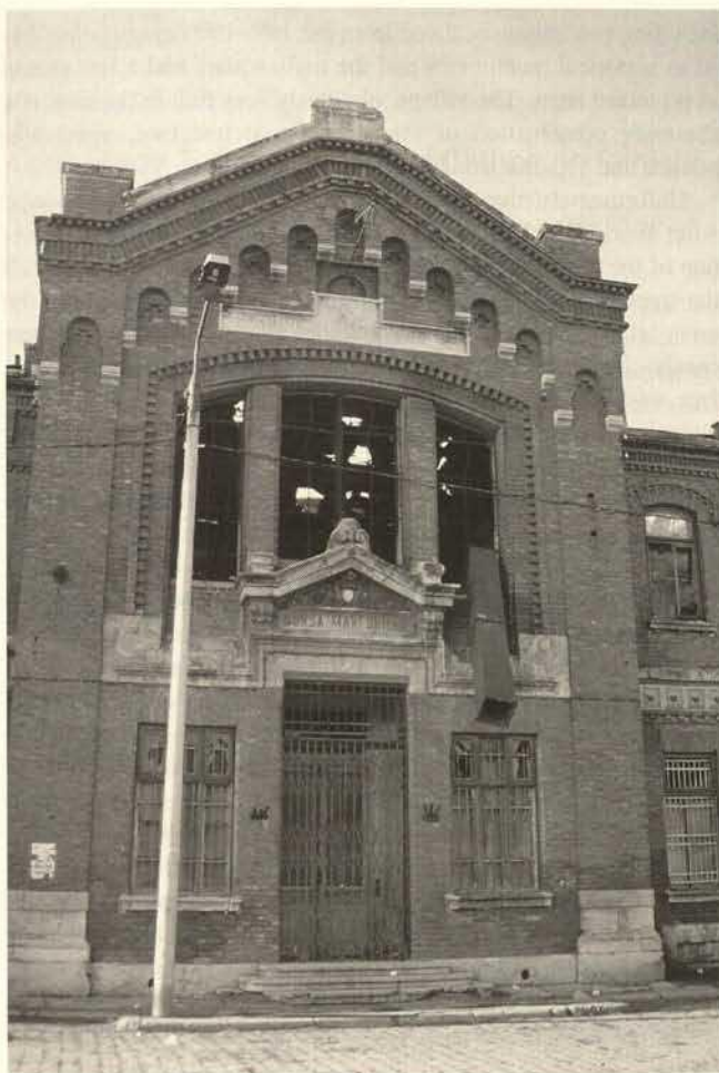
Bucharest's merchandise control point, built in 1900 by the Italian architect Giulio Magni, has been abandoned since the fire that seriously damaged it in 1992.
