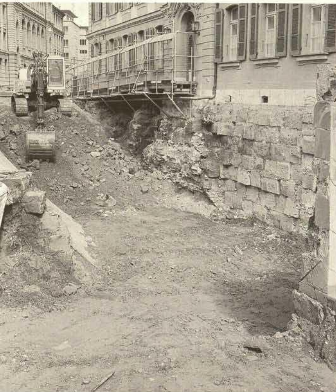
Bern, Waisenhausplatz. The excavation pit for the underground car park goes right up to the walls of the Waisenhaus.
