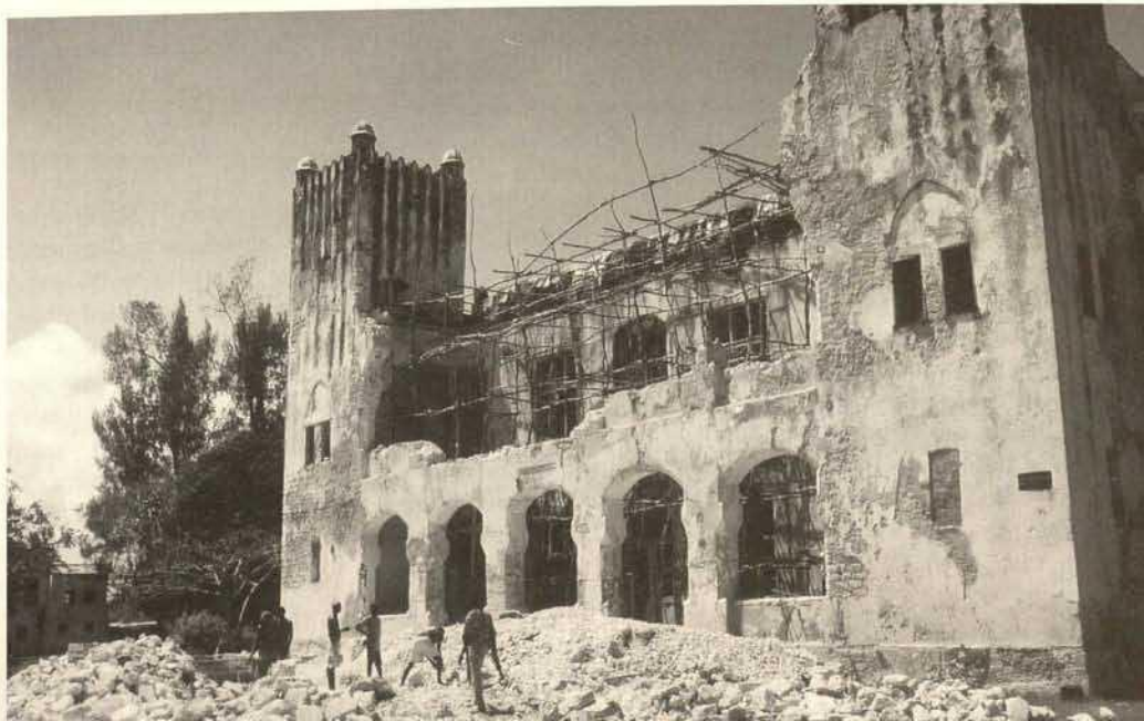
The Boma after December 2000: dangerous parts of the façade had to be taken down. Will it be possible to reconstruct it soon?
