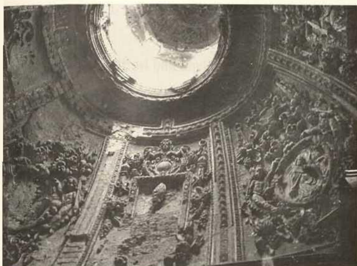
Palace chapel in Berezhan, detail of the stucco work in the cupola
