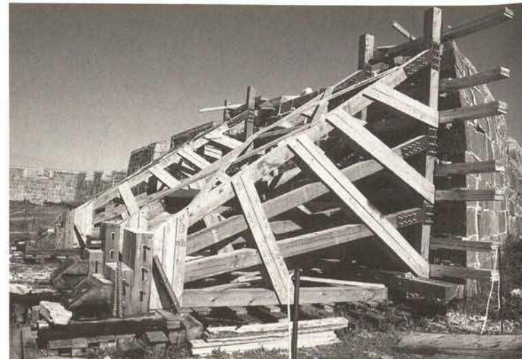
Shoring, Point of the North-West bastion, Fort Prince of Wales, Churchill, Manitoba
