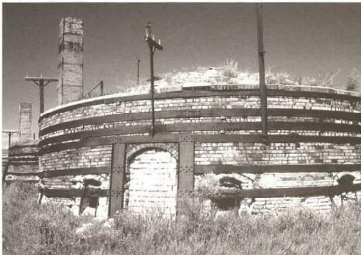
Typical deterioration, Kiln No 5, Claybank Brick Plant, national historic site, Claybank, Saskatchewan
