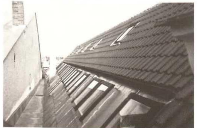
Telč: inappropriate alterations to the roof of one of the most valuable historic houses at the square
