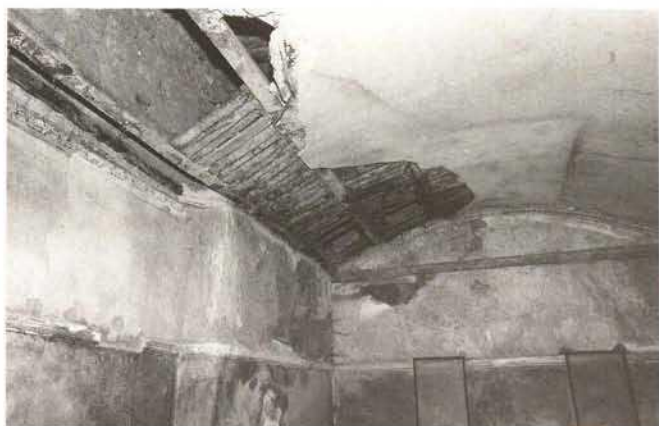
A lack of care taken during conservation measures leads to the decay of formerly well-preserved wall paintings. The barrel-shaped vault with its precious wall paintings, almost completely preserved 90 years ago, has collapsed due to a gap in the protective roof. Rapid deterioration is the consequence.
