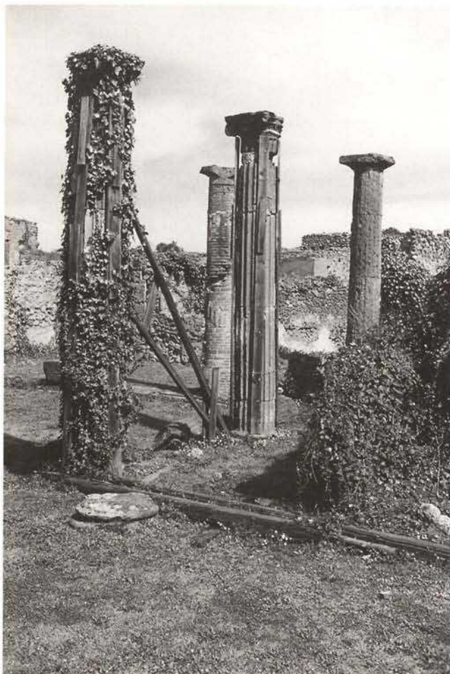
Scanty, temporary conservation measure bracing the columns of a peristyle house. After the earthquake of 1980 endangered houses and constructions were provisionally secured. After 20 years the temporary solutions are still in place, but have corroded or are slowly decaying, since the necessary measures have never been taken. Ivy growth is accelerating the process of decay.
