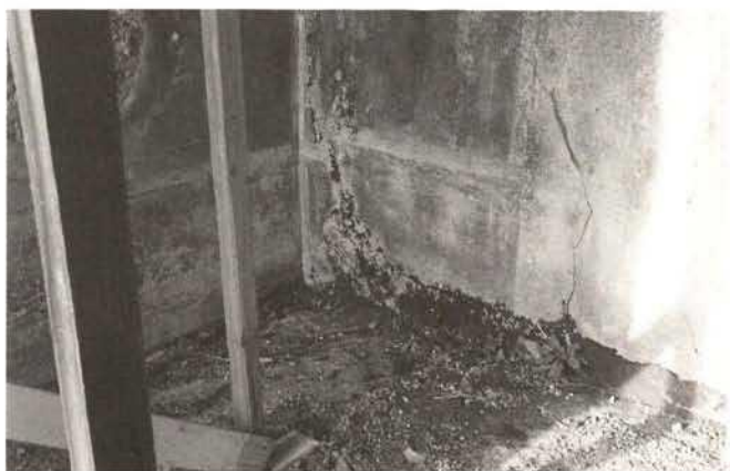
Destruction of the wall painting by moss.
