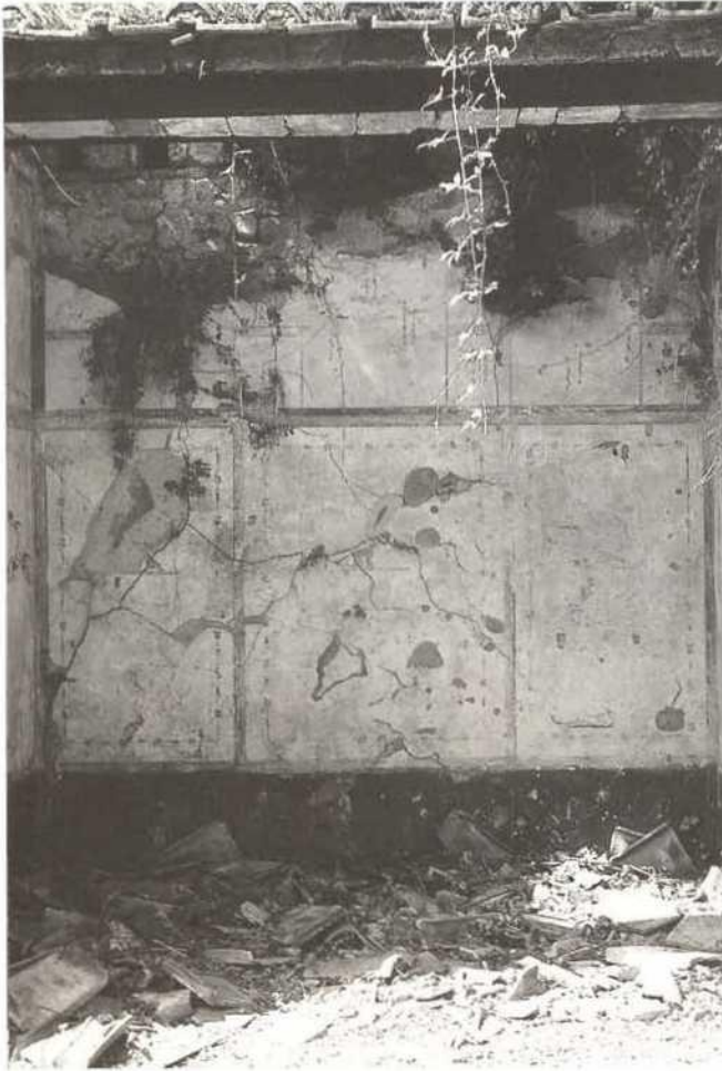
Room in a state of complete neglect, with interior wall painting already severely faded (Casa di Ifigenia).
