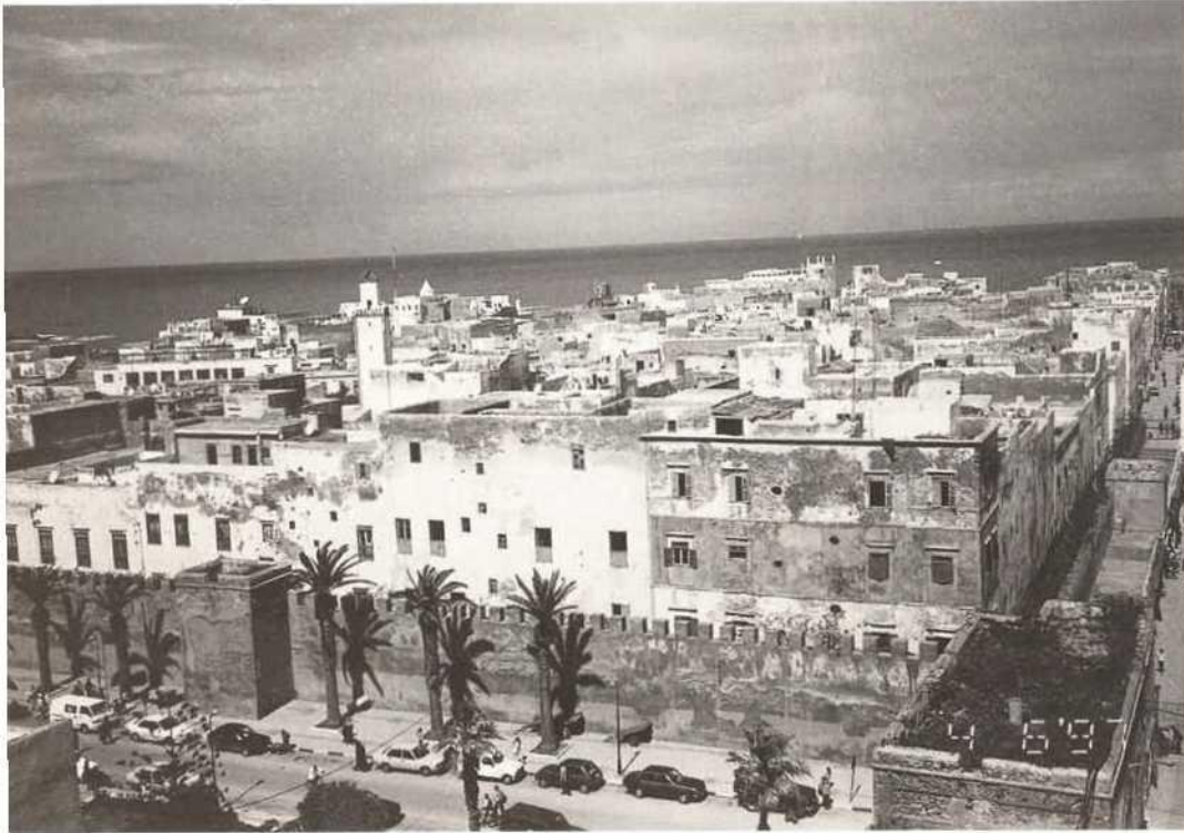
Essaouira (Mogador). Second east wall: rising damp due to surface water and rain water, causing stone surface erosion
