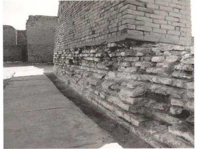
Moenjodaro, saltpeter in a burnt brick wall, lower city
