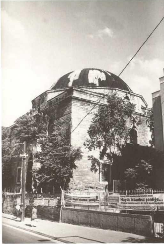
Bath of Bayezit is an early 16 th century building which has not been in use for many years. During the road-widening operation in the 1950's, the street level was changed and the foundations of the south wall were exposed. A crack which had developed earlier on the dome of the dressing hall was widened by the tremors in 1999.
