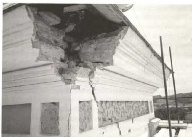
Mionica, part of church tower damaged by earthquake
