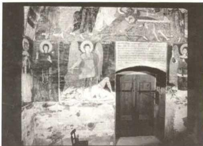
Bodjani, fresco painting damaged by humidity
