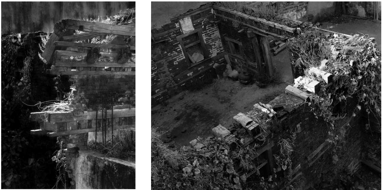
Fig. 9 and 10 Views of ruins of a house in the walled city of Ahmedabad, showing a form of timber lacing similar to that found in taq construction in Kashmir. In the partially dismantled building, the construction with runner beams tied together with cross-timbers pegged to the beams is visible (photographs © Randolph Langenbach)
