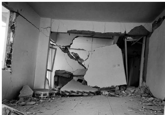
Fig. 13 Collapse of a brittle interior hollow clay block wall illustrating typical failure pattern for such walls lacking subdivision of the masonry (photograph © Randolph Langenbach)
