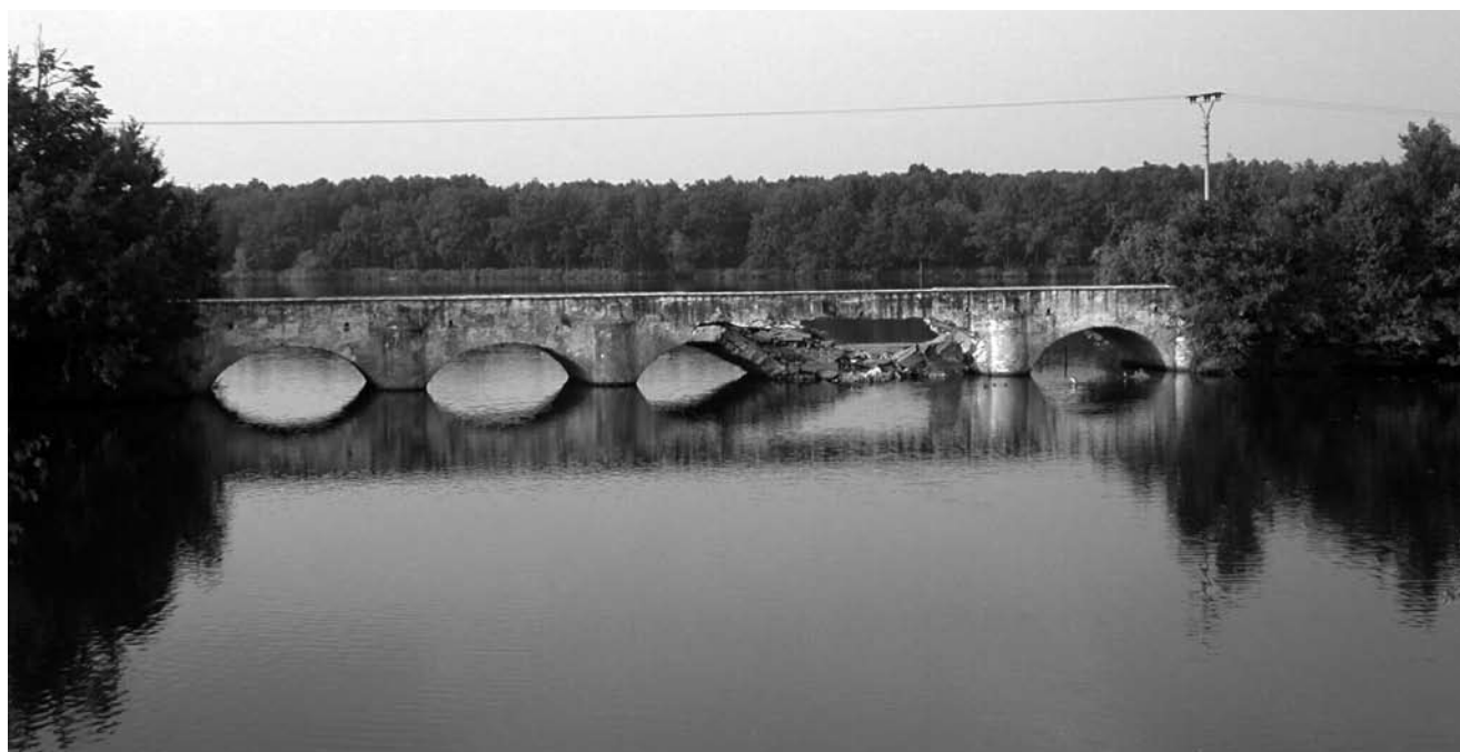
Fig. 4 Stará Hlína, the Inundation Bridge, a masonry bridge from 1781, historically located in the Třeboň pond system. Part of the bridge collapsed; it is necessary to reconstruct the bridge pillar as well as two bridge spans.
