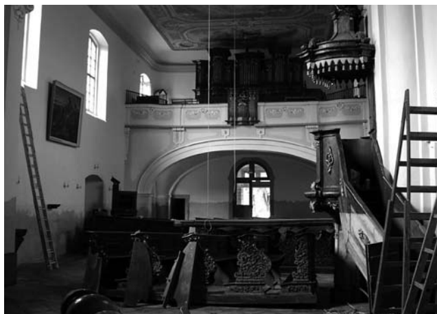
Fig. 10 Štětí, area of St. Simon and Juda Church, 1785. Church foundations at the sidewall were undermined; plasterwork, stone components and movable objects are damaged.
