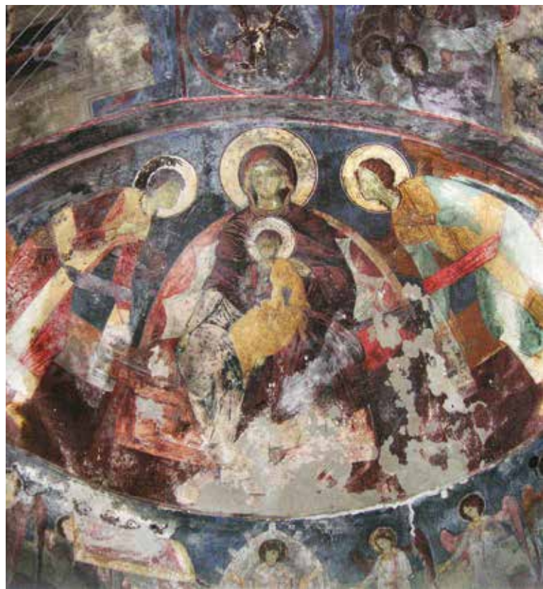
St. Nicolas Church, abrasion and loss of preparation and paint layers
