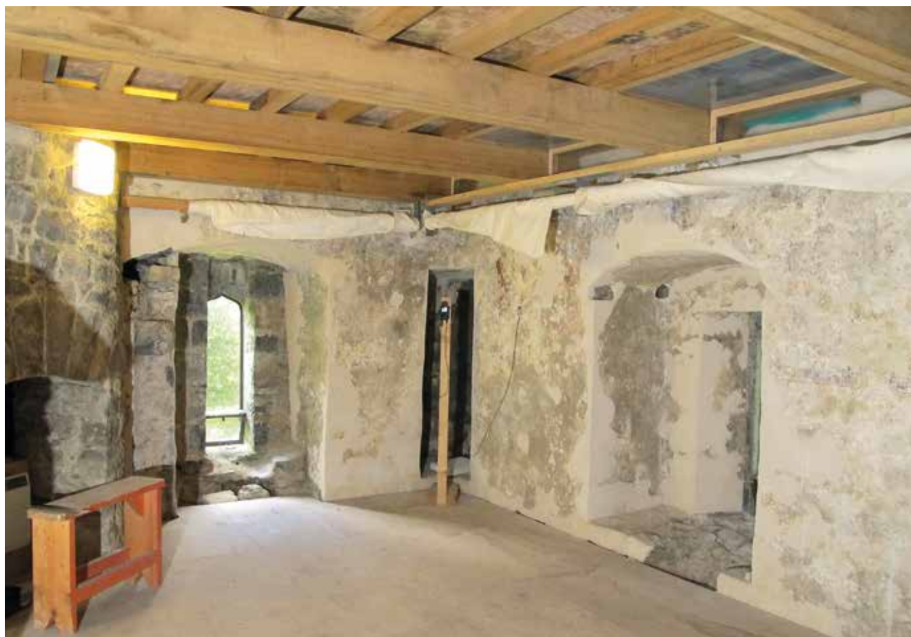
Ardamullivan Castle, with curtains rolled up the situation becomes visible as immediately after the conservation. The ceiling is new and unnecessary; the electric heating even dangerous. What is still missing, is at least a minimal presentation of the wall-paintings.
