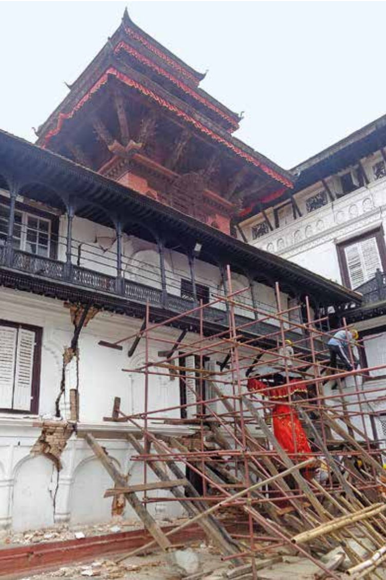
Shoring to protect the façade from collapsing onto the main Hanuman Statue with the intact Agamchhen Temple that is raised on timber stilts over the palace
