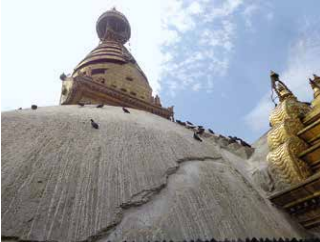
The Swayambhu Mahachaitya showing the temporarily sealed cracks after removal of layers of lime-wash
