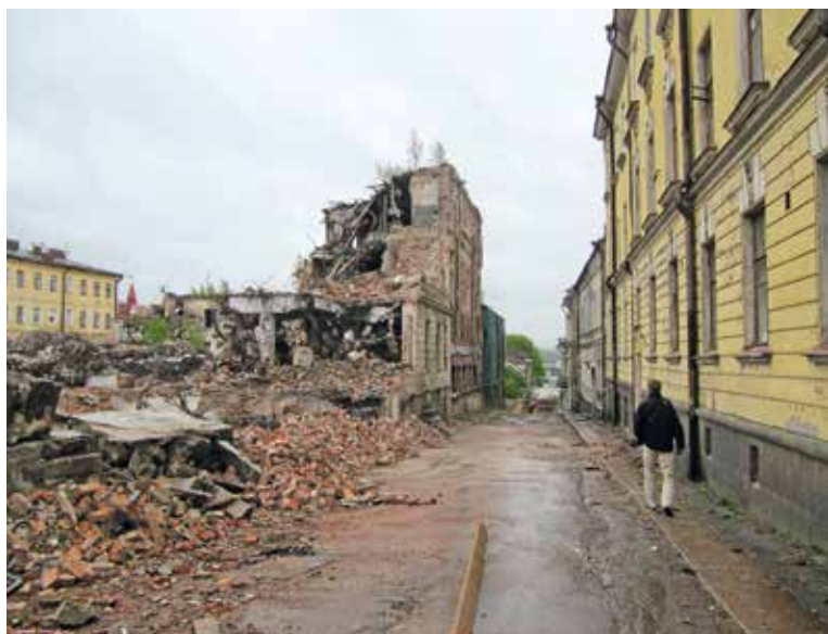
Demolished block in the middle of the town (photo Maija Kairamo, April 2013)
