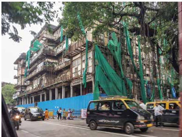
Fig. 10: Esplanade Mansion, barricading and provision for pedestrian pathway by MHADA after Court Orders, July 5, 2019
