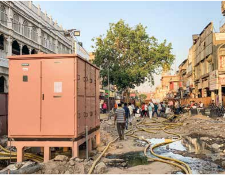
Fig. 7: Current view of transformers being installed on the central median where the historic canal flowed (photo Smita Datta Makhija, October 2019)
