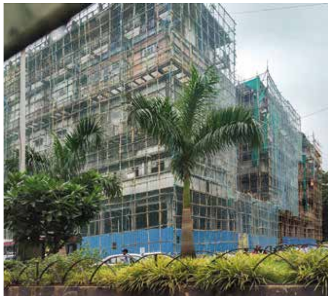
Fig. 11: Esplanade Mansion, protection and netting done by MHADA after Court Orders, July 23, 2019
