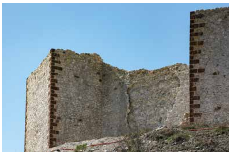
Fig. 5: The collapse of walls after interventions (photo C. Jäger Klein, 2019)
