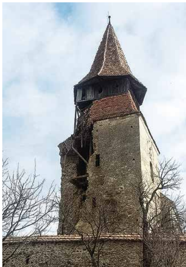
Fig. 2: The church tower of Roades after the collapse (photo A. Schnell, 2016)
