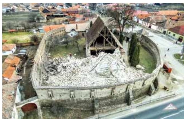
Fig. 4: The church in Rotbav after the collapse of the tower (© www.honigberger.com, Christian Chelu)
