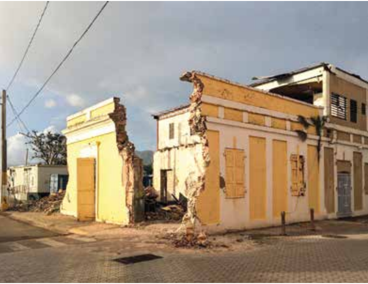
Fig. 4: Puerto Rico, house destroyed by a hurricane in 2017 (© Parala Naturaleza)
