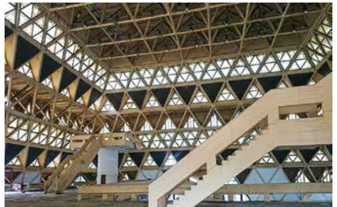
Fig. 7: Interiors of Hall of Nations showing the system of natural lighting, sound state of materials and structure (© Kiran Joshi, September 2016)
