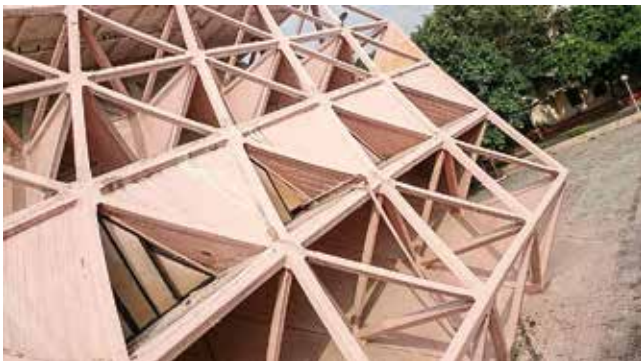
Fig. 5: Hall of Industries conceived as a combination of four square pavilions with chamfered corners (© Kiran Joshi, personal collection, September 2016)
