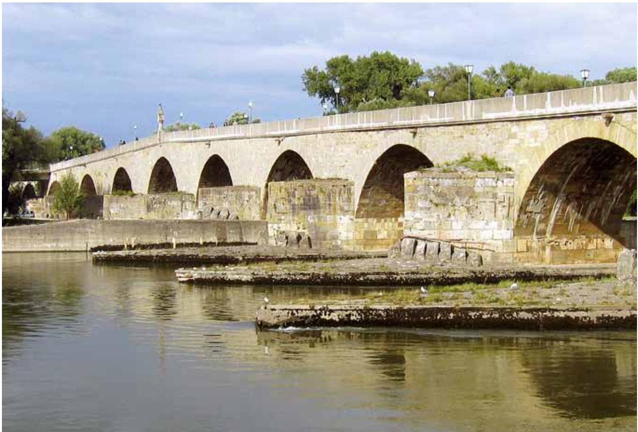
Fig. 2: Protection of bridge piers' foundations against undermining by means of small islets with a paved upper surface – a historical example in Regensburg (Bavaria)
