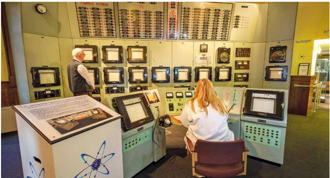
Fig. 4: DMTR control room in Caithness Horizons.
