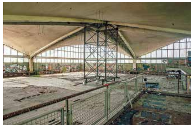
Fig. 11: Multi-purpose hall in Magdeburg (built 1969); endangered structure of four hypar shells, with temporary support in the centre (© Sebastian Schmidt)
