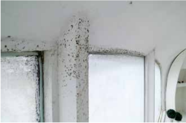
Fig. 12: Inside the deck before restoration (2015): frozen condensation on the windows, water and mould on the concrete shell (© adb Ewerien und Obermann)
