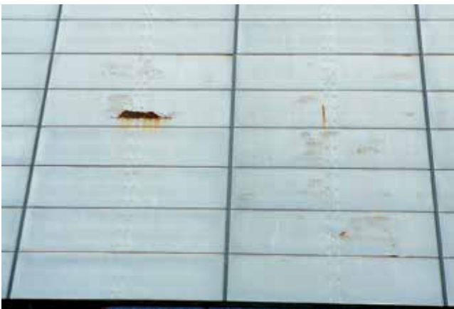
Fig. 4: Sandwich panels with faded coating and corrosion, 2013 (© adb Ewerien und Obermann)
