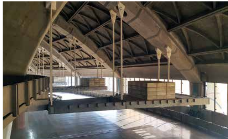
Fig. 4 Interior view of the Stadium circulations showing the innovative structural system of prefabricated-concrete cantilevered consoles
