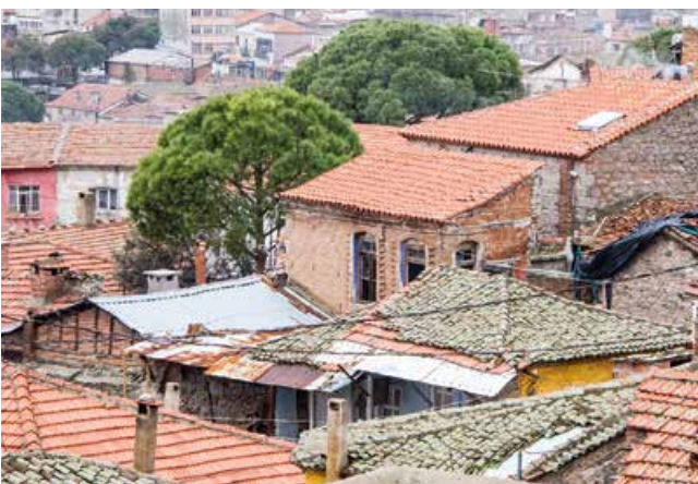
Fig. 5: Maintained roofs can protect houses in longer terms, while neglected roofs instantly transfer the decay (Photo: DAI-Pergamon Excavation, Ulrich Mania)
