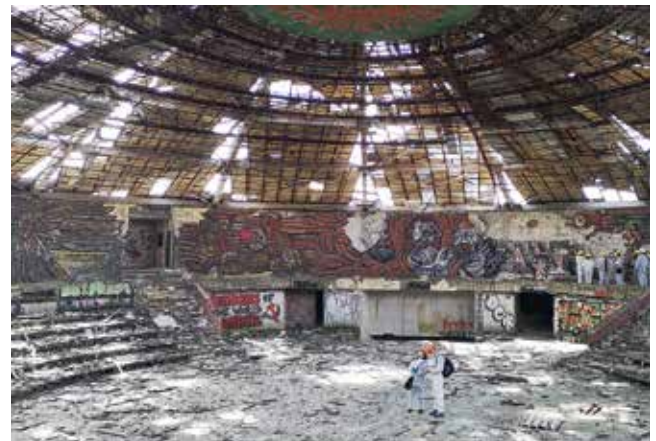
Fig. 9 The interior of the main hall where the inner mosaic ring and the steel roof structure can be seen
