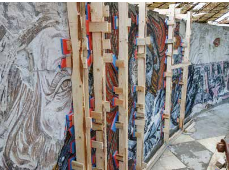
Fig. 8 Main Hall, inner ring, detail of the head of Marx after the left side of the face fell off and during mechanical securing of the hollow mosaic, September 2019
