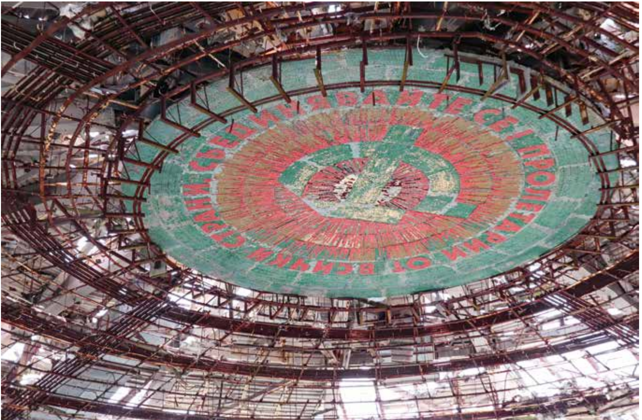
Fig. 2 Interior of the monument in disrepair
