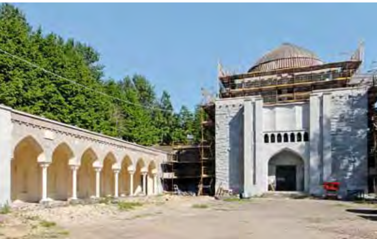
Fig. 5 Restoration of the House of Ablution in the Jewish cemetery of St Petersburg, 2011 (Photo: Pavel Platonov)
