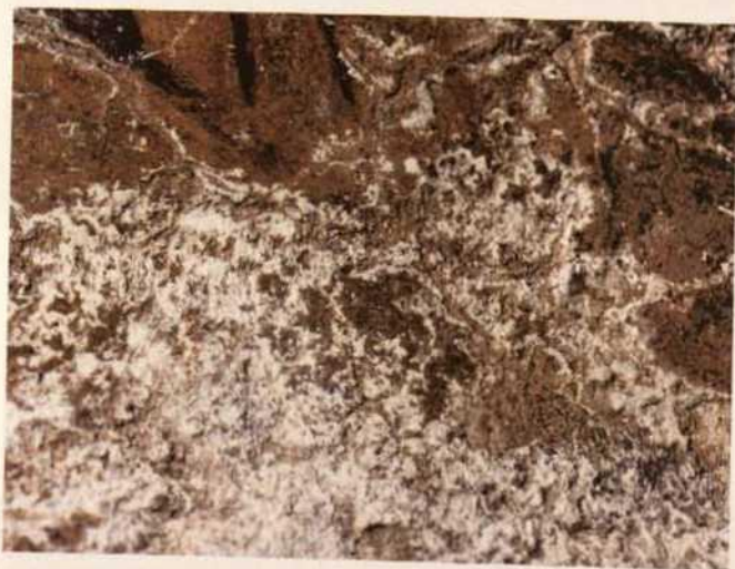
Fig. 18. Ston, Church of St Michael, wall paintings (see fig. 17), detail: salt incrustation.
