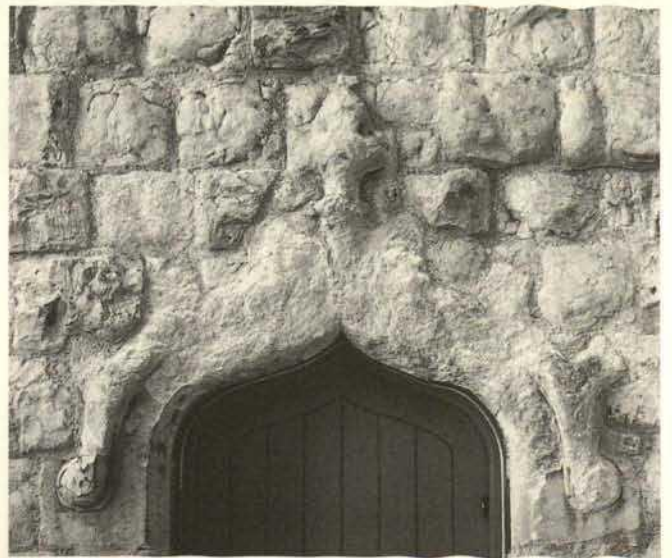
Fig. 5. Remnants of Hood Mould over Door. – Different approaches are possible within the Society’s philosophy of conservative repair. The severely decayed hood mould over the door is an eloquent reminder of the building’s history, and could be left alone (as has happened). On the other hand it could be argued that for technical reasons, but no other, it is important to renew it to allow it to shed rainwater.
