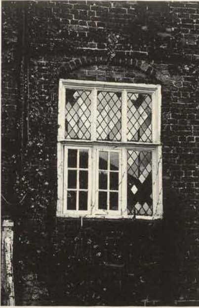
Fig. 3. Alterations to Window. – The insertion of wooden casements in part of this 16 th window, perhaps 150 years ago, adds to its interest and evoking history, and should not be removed simply on the grounds of “correctness” or “tidiness”.
