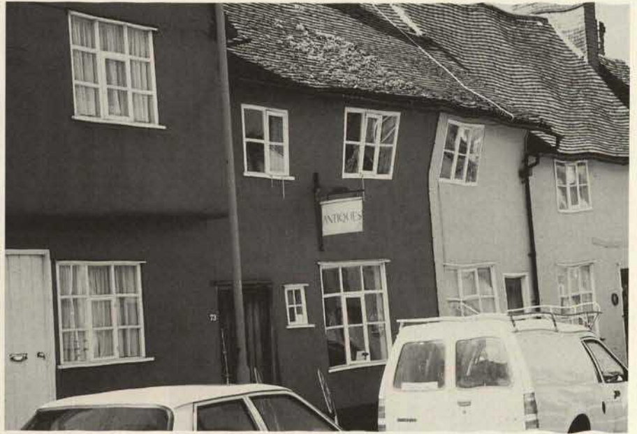
Fig. 4. Old Structural Movement ... – All old buildings move, like this timber framed one. This is part of its character. In Britain too much effort is spent on trying to correct movement that may have stopped hundreds of years ago, or on remedying faults that have to be misunderstood.
