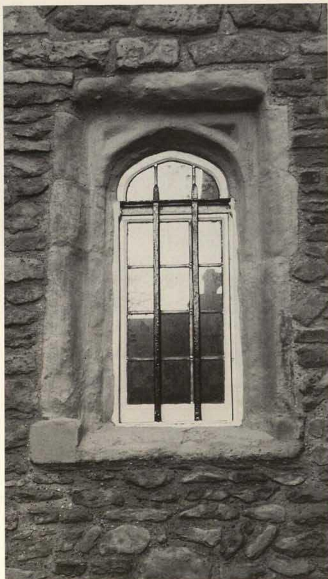
Fig. 6. Lime Conservation. – The use of a lime and stone dust “shelter coat” has protected this Mediaeval stone window, and avoided the need to replace it or use a modern chemical consolidant.
