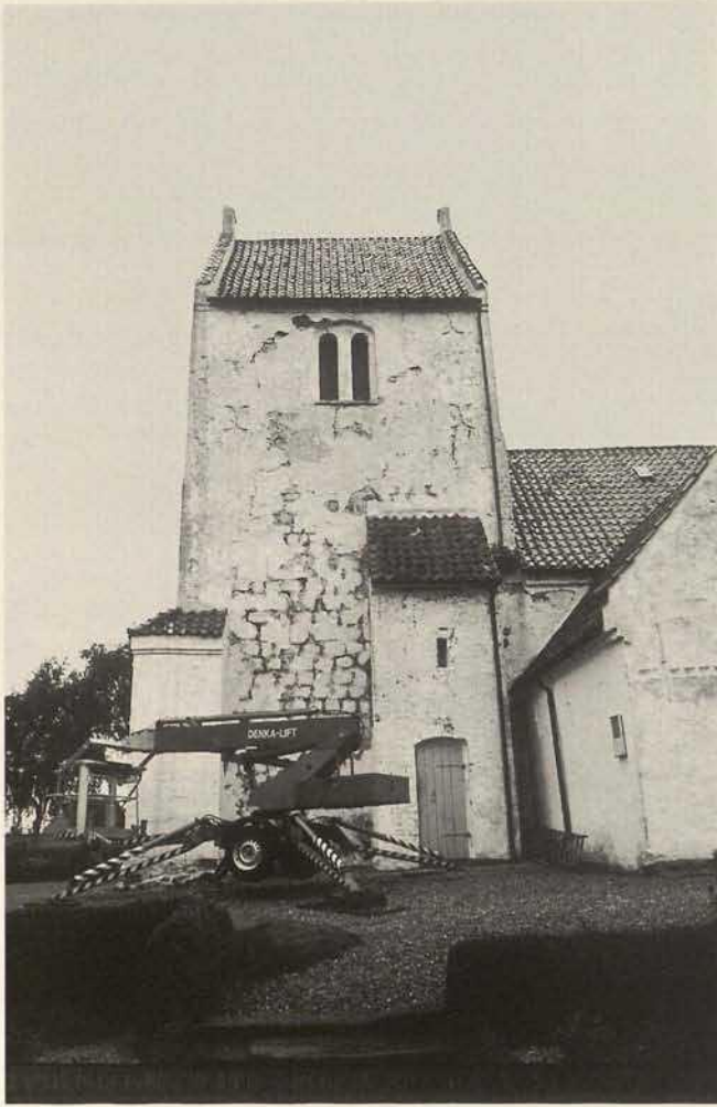
Fig. 5. Vallekilde Church (Zealand). The tower after cleaning in 1991. The lower part is made of granite boulders and the rest partly of hard-burnt bricks. In those areas, a cement slurry was preserved.
