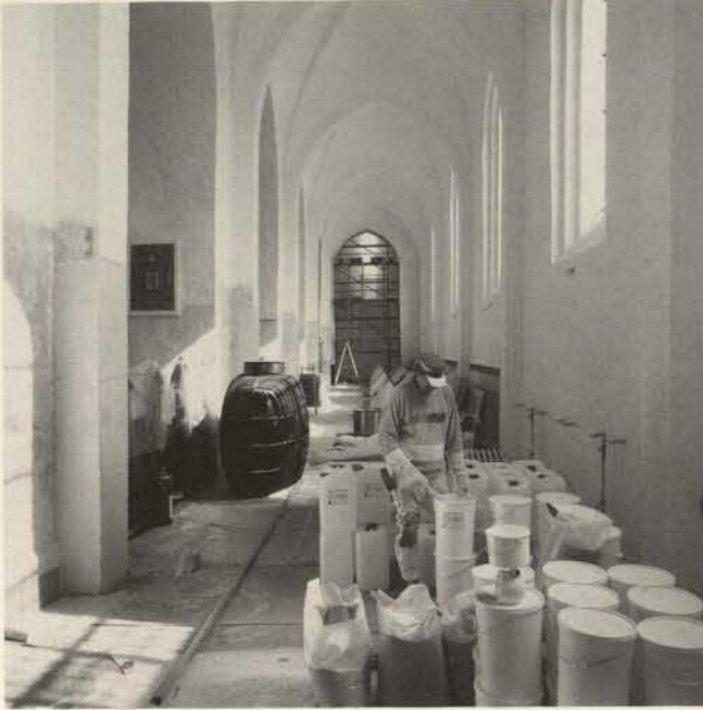
Fig. 2. Lime putty, quartz sand and limewater delivered ready for lime-washing the cathedral in Århus.
