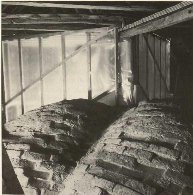
Fig. 8. Kirkerup Church (Zealand). The top side of a 14th century vault, with bricks showing deterioration caused by salts (mostly natrium chlorides).
