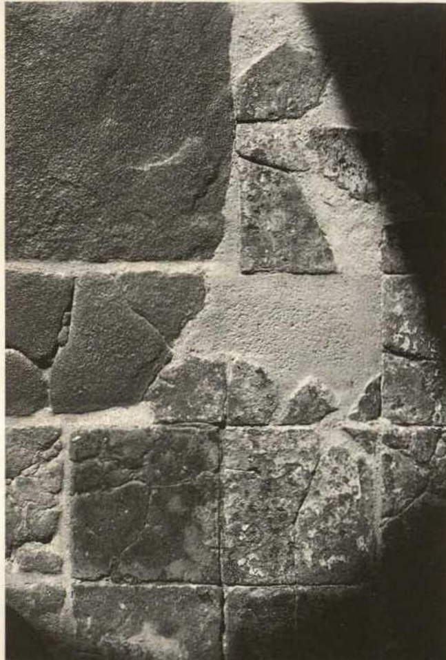
Fig. 13. Fourth case study: Acton Court. Cross passage floor on completion of lime repairs. Note area of contrasting mortar to indicate resiting of buried tiles.
