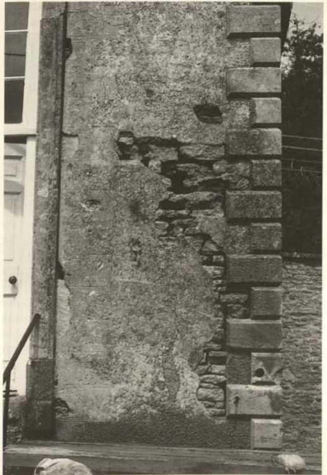
Fig. 1. First case study: Church House Gazebo. Preparation for lime mortar consolidation and lime roughcast render. Loose material was associated with settlement in the structure.
