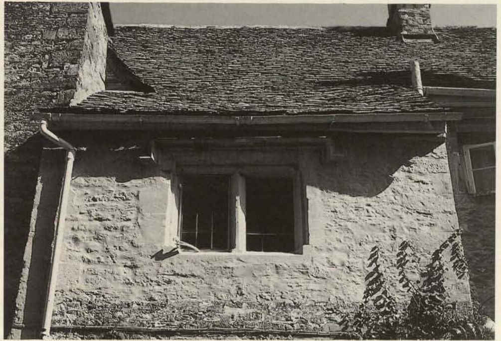
Fig. 7. Second case study: Woolgatherers staircase. Completed lime repairs to mortar joints and stones, and five coats of limewash.
