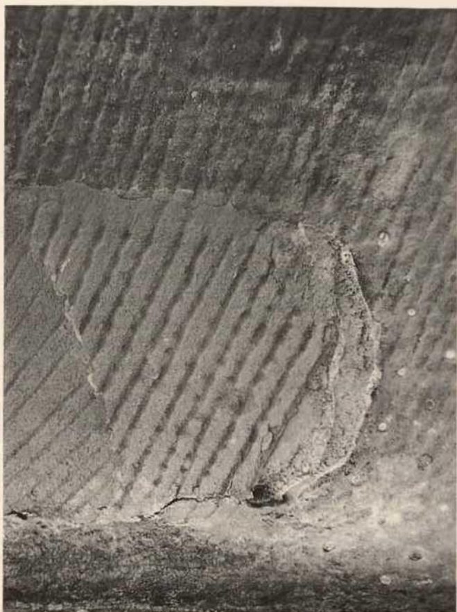
Abb. 12. Salzschäden am Randantrag einer Reparaturstelle Fig. 12. Damages caused by salts at the application rim of a repair area
