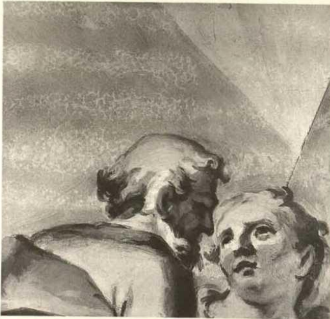
Fig. 9. East chapel next to the choir arch; damages from penetration of condensation moisture in cracks caused by shrinkage
