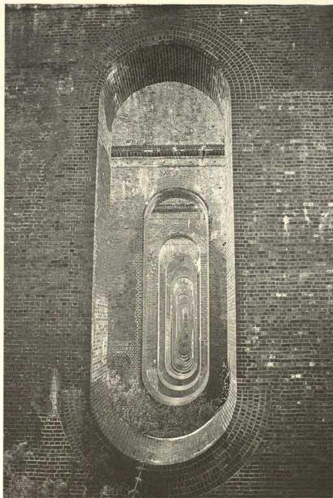
Ill. 7. Balcombe viaduct on the London to Brighton line is a monumental Italianate structure with a spectacular enfilade of arches in the piers.
