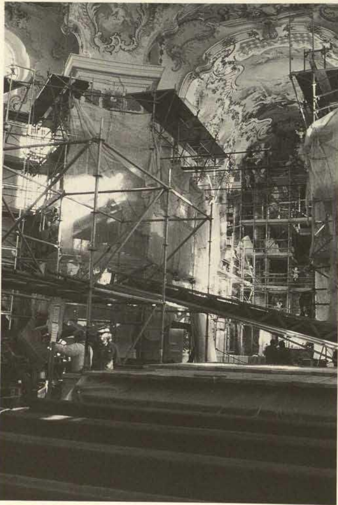
Blick zum Chor, während der Restaurierung 1990 View toward the choir, during restoration in 1990
