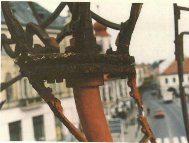
3a, b. Prague, equestrian statue of Jiri z Podebrad (J. Schnirch, 1890); corrosion damage of inner iron skeleton
