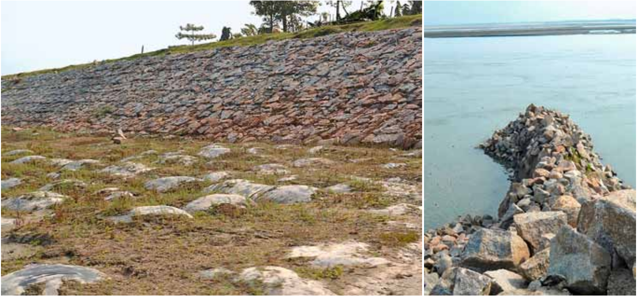
Fig. 6: Stone Spur before & after the floods of 2013
