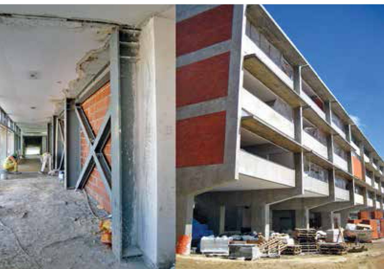
Fig. 10: Padre António Vieira High School, Ruy Athouguia, 1959–1964; Teresa Nunes da Ponte, structural reinforcement, 2009
