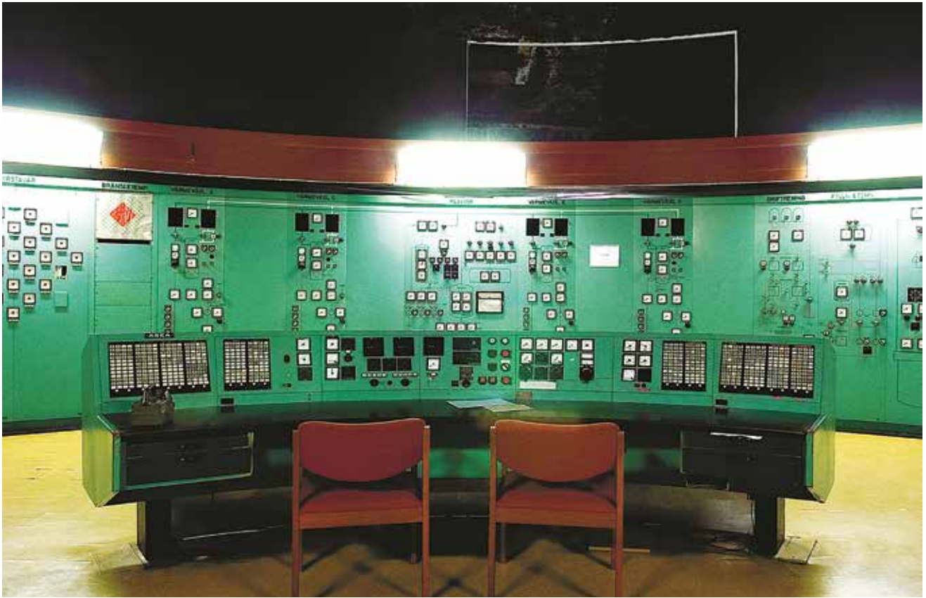
Fig. 8: The Control Room is situated in a separate cavern within the rock, connected to the reactor hall by airlocks. The Control Room allowed supervision of the entire plant from one place.
